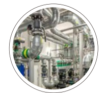
Fan and Water pump
